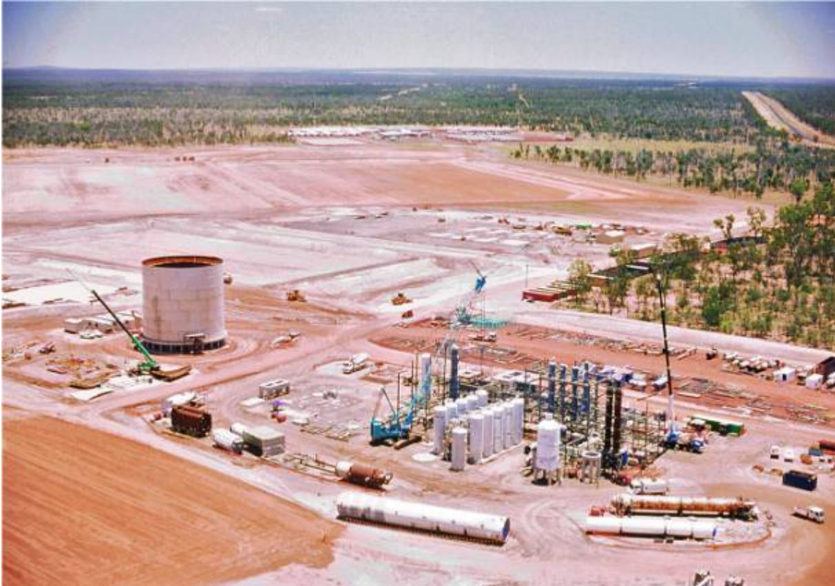
Re-construction of the ammonia plant and new ammonia tank, with power plant, evaporation ponds and camp site in background (late 2007)
